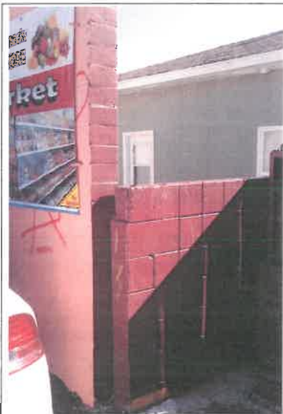
Wall with Graffiti Partially Covered by El Super Banner
