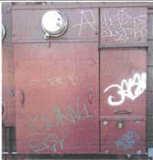
Graffiti on North Side of Laundromat Exterior Wall and Electrical Box
