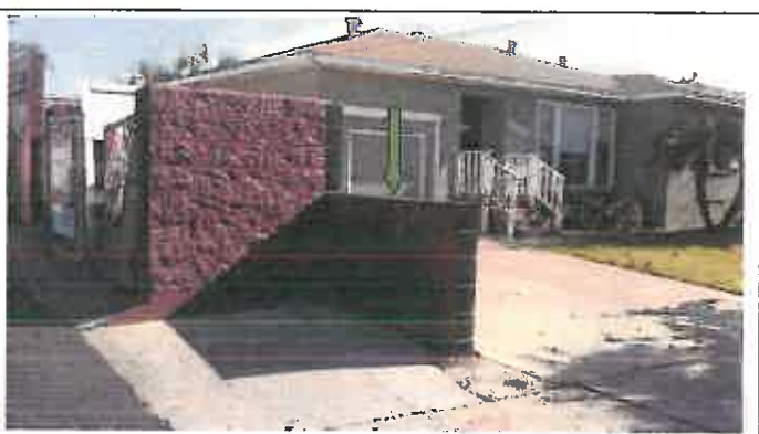
Graffiti on Wall and Broken Glass Separating Business from Residences
