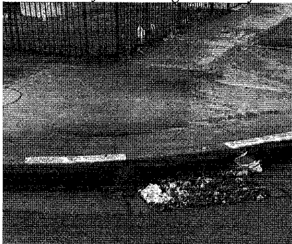
Picture 3: City drain being blocked by trash
