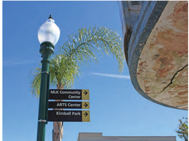
Directional sign mounted on street light
