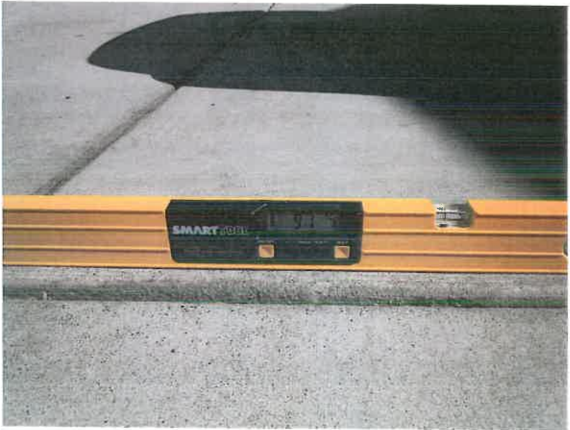
Close-up of Smart Level at Driveway of 3108 E. Division Street with slope reading of 9.1% (looking east)
